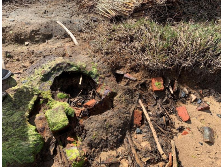
Figure 14: Rubble, debris and undercut sedge adjacent to Chester Rd revetment
