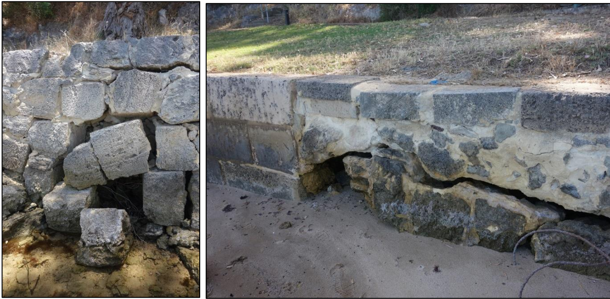
Figure 9-19: Some Examples of Walling in SRPep01 Requiring Maintenance (Jan. 2015)
