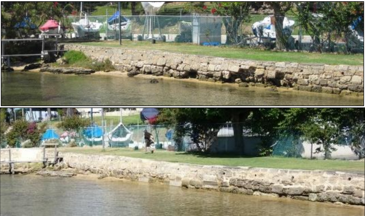
Figure 9-11: Example of SRPep02 Walling Failure and Maintenance (2010 Top, 2014 Base)
