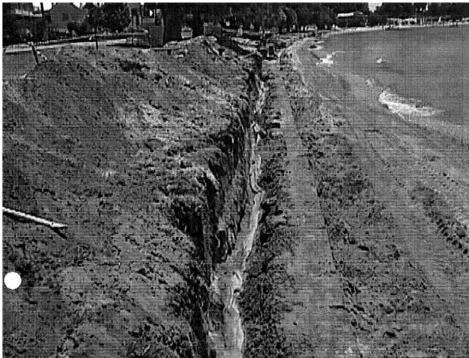
Figure 10-5: December 2001. Reconstruction of walled section between Mosmans and 185m walled section replaced in 2001 (SRT 2001)
