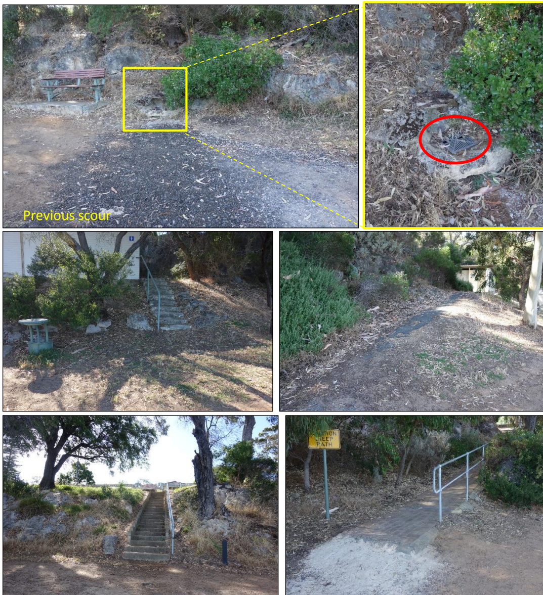
Figure 9-20: Examples of Unmanaged Surface Runoff in SRPep01 (Jan. 2015)
