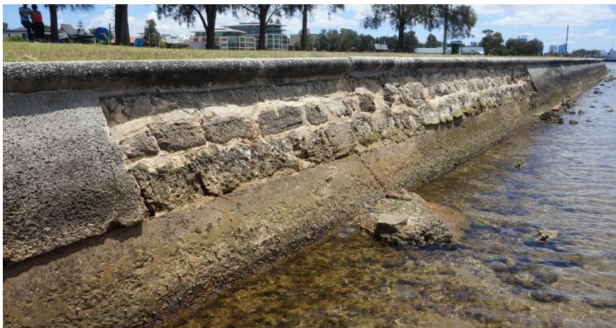
Figure 7-11: Inclined limestone block walling north of NYC with concrete panels on old footings
